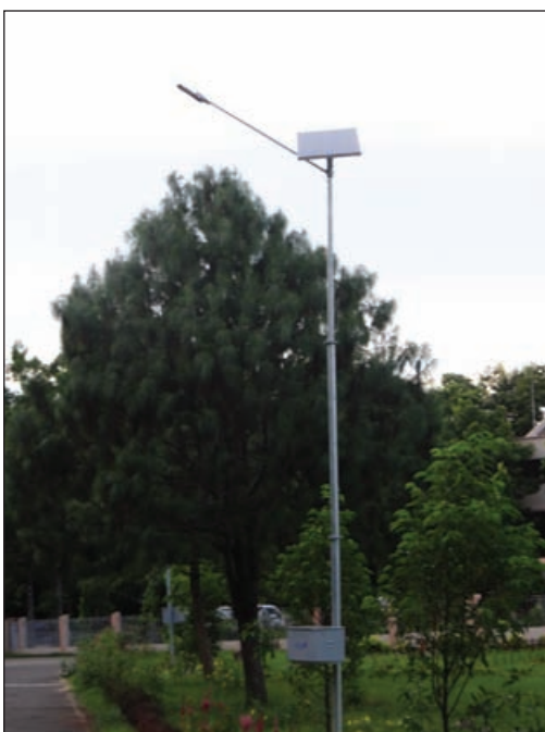
Solar Street Light
